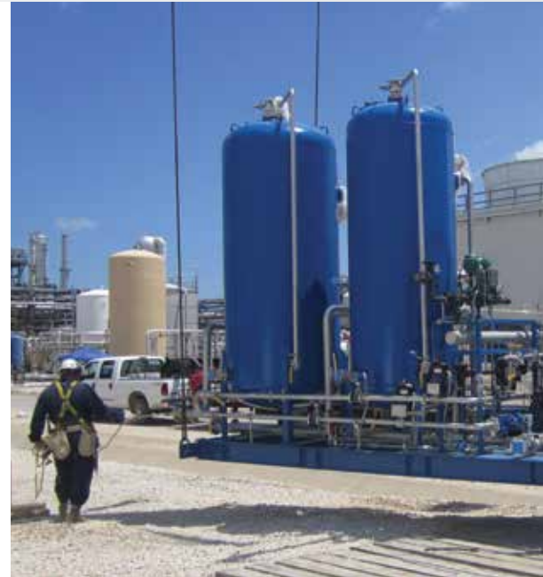
Culligan® custom designed counter current, automatic demineralizer system built for Texas Chemical plant for process and boiler feed water.
